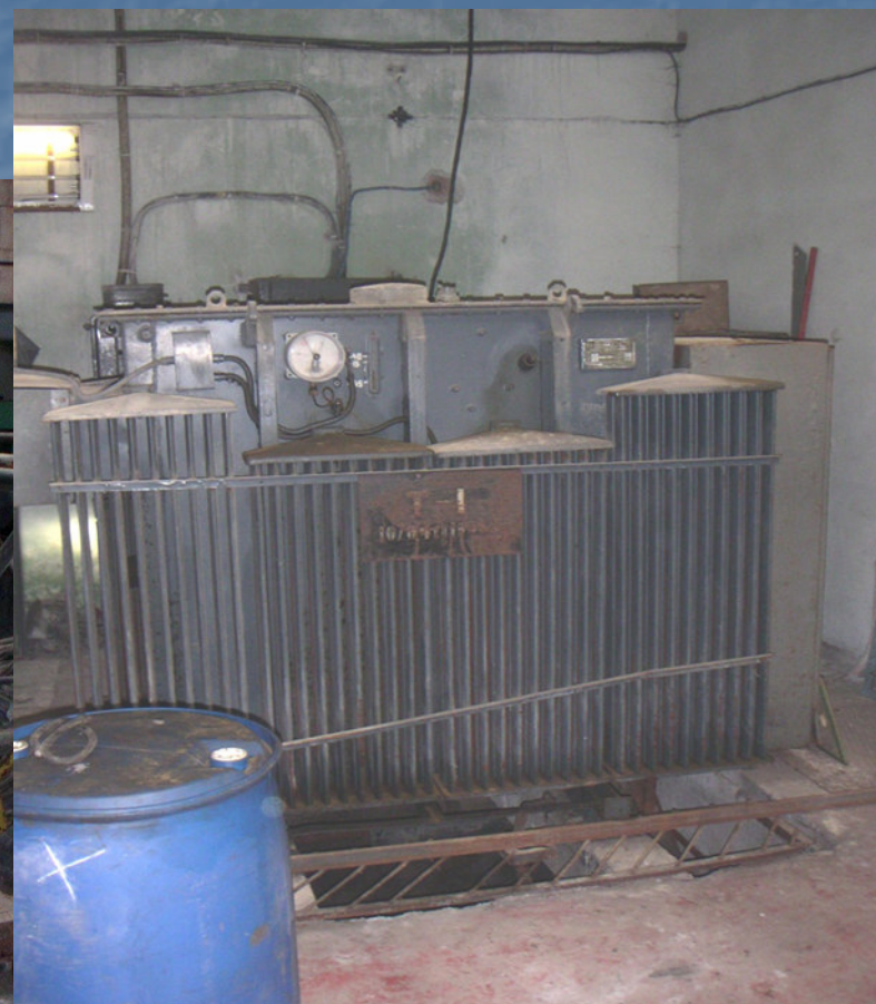
PHB saturošs transformators
